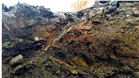
While repairing an irrigation line, Randy Dowdy found jumbled soil deposition. "Even the soil that was saved and put back on my land wasn't segregated."
