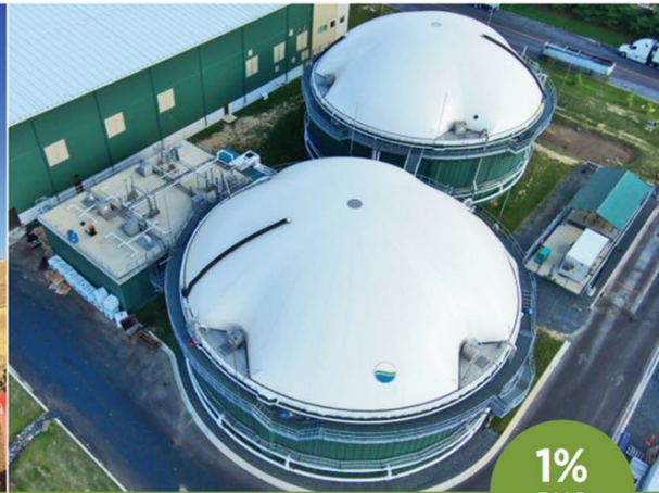
Bioenergy Devco RNG | Jessup, Maryland
